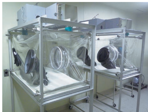
Figure 5. Vinyl isolators in the quarantine room
